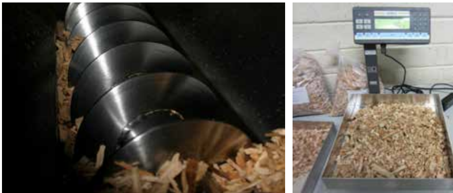
Figure 4: Panel A shows a wood chip auger infed to an industrial biomass boiler for steam production. Panel B shows part of the routine quality testing procedures employed to ensure the quality parameters of supply lots. Variation in quality parameters (moisture and others) can be high so processing plants rely greatly on the knowledge and experience of contractors to help ensure that a consistently high quality product is supplied.
