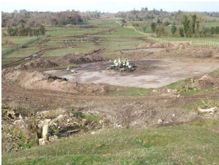
Figure 1: Excavation in progress showing the type of landscape the M6 traverses (NRA).
